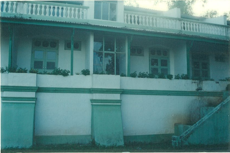
The back of the building with heavy buttresses. The verandahs face the sea
