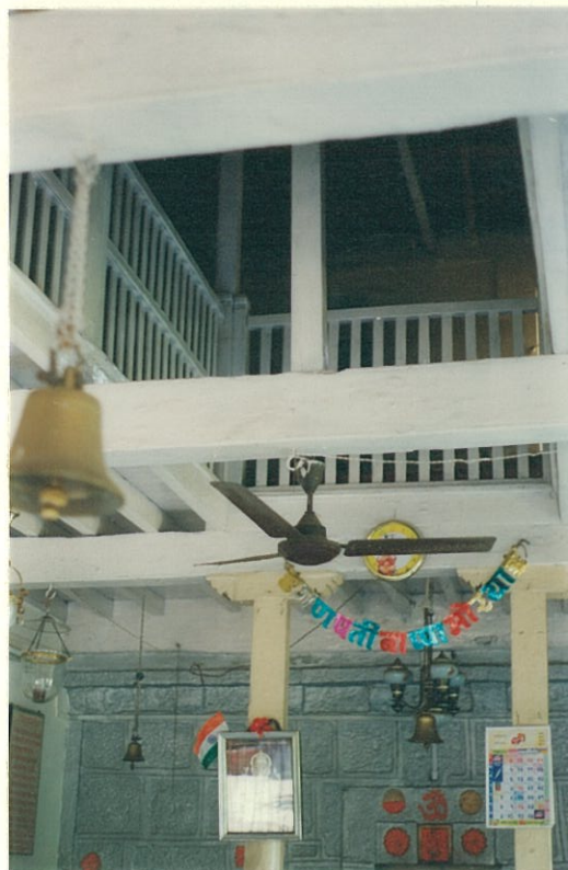
Interior view showing TW mezzanine, all around a central cut out, supported over bracketed timber columns
