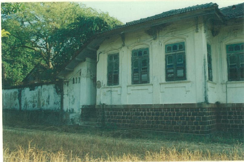
Side view of the building showing articulated bays and a high stone plinth
